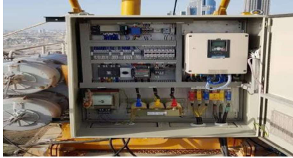
Gambar 2. 4 Panel kontrol Crane
