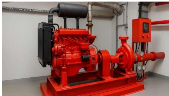
Gambar 2.5 : Emergency Fire Pump
