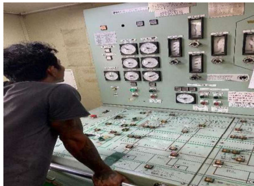
Gambar 2.5 : Ballast Control Room
