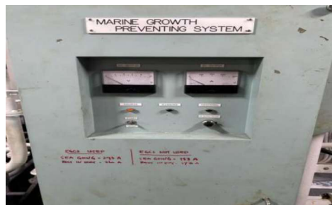
Gambar 2.7 Power Supply Unit
