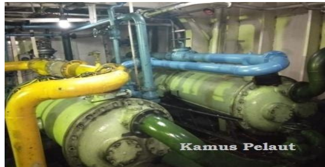
Gambar 2.13 Sea Water dan Fresh Water Cooler
