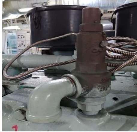
Gambar 2. 7 Safety Valve Sumber: Dokumen Penelitian
