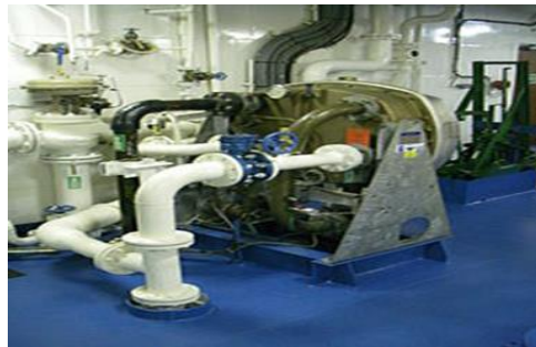
Gambar 2. 1 Fresh Water Generator
