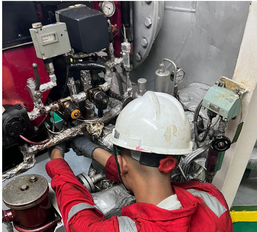
Gambar 4. 3 Pengecekan safety device burner Sumber : Dokumentasi pribadi (2021)
