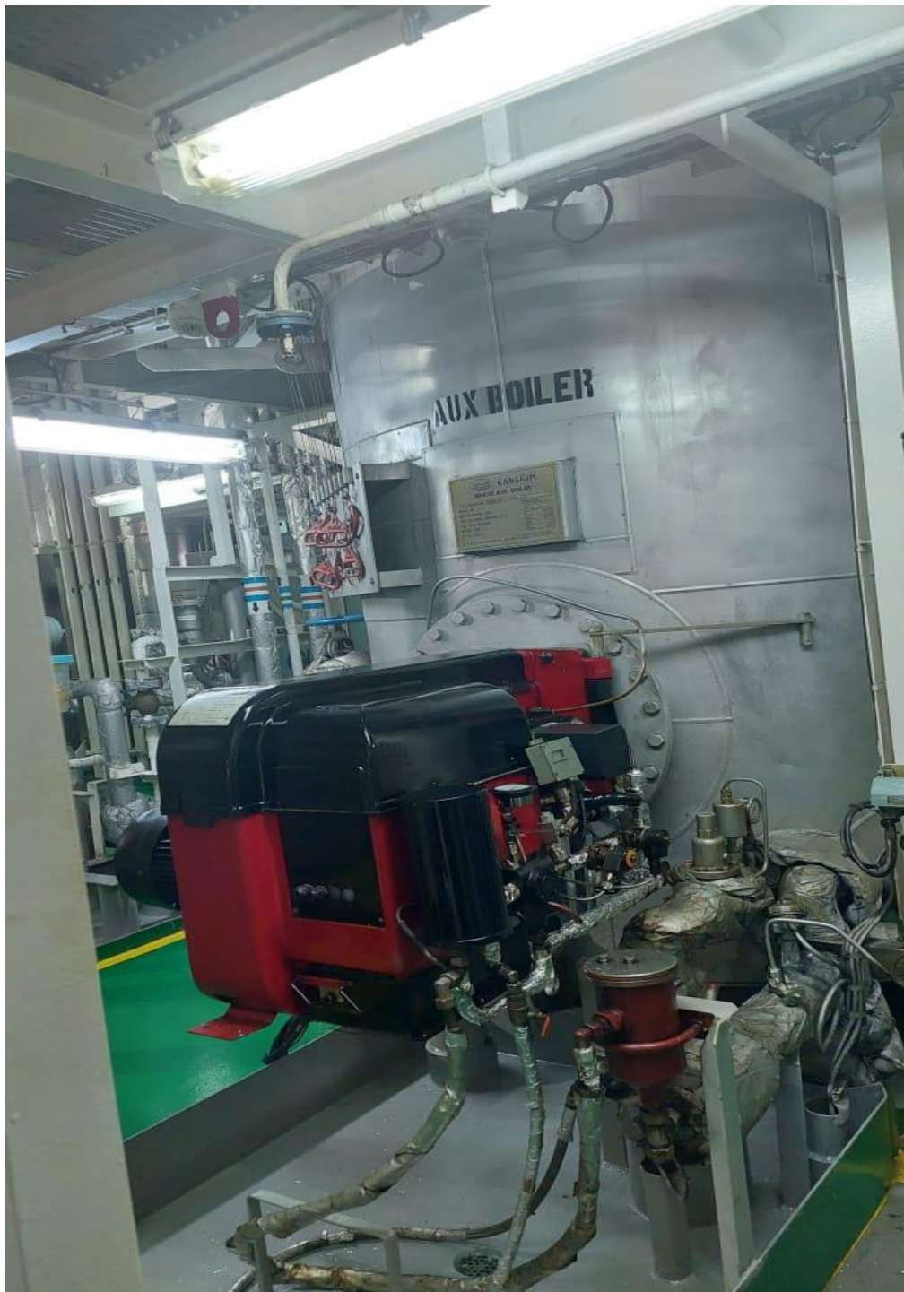
Lampiran 10 Auxiliary Boiler
