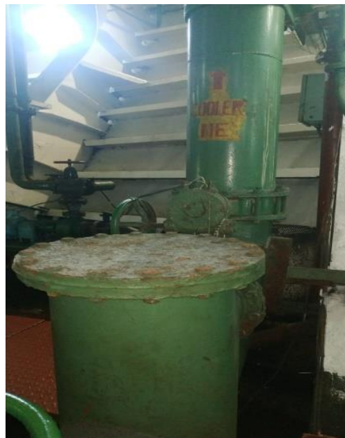
Gambar 2. 10 Sea Water Cooling Pipe
