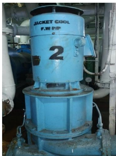
Gambar 2. 2 Fresh Water Cooling Pump
