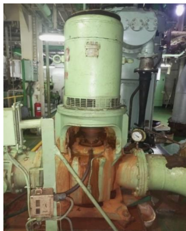
Gambar 2. 8 Sea Water Cooling Pump
