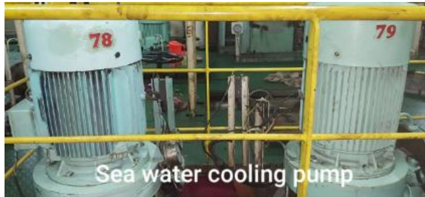
Gambar 2.24 Sea Water Cooling Pump
