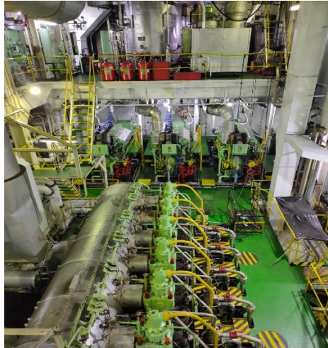
Gambar 2. 3 Ruang Kamar Mesin MV. NAMEERA
