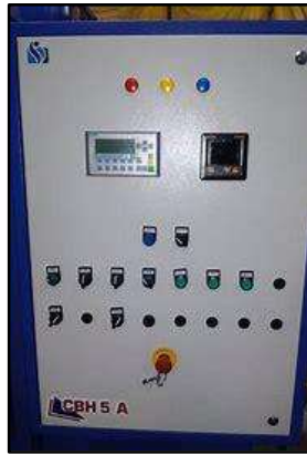
Gambar 2. 5 Automatic Control Panel
