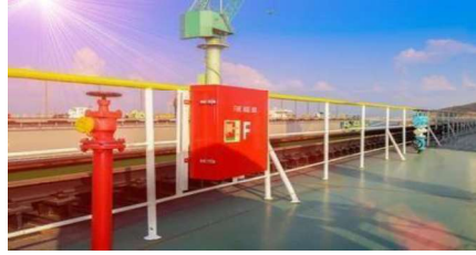
Gambar 2. 7 Outdoor fire hydrant
