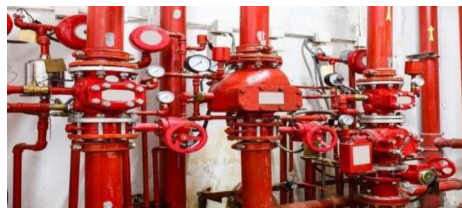
Gambar 2. 2 Fire Main Pipe
