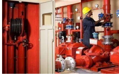
Gambar 2. 6 Indoor Fire Hydrant
