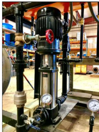
Gambar 2. 20. Feed Water Pump
