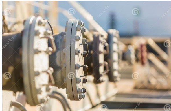
Gambar 2. 7 Manifold Sumber: china-industrialhose.com
