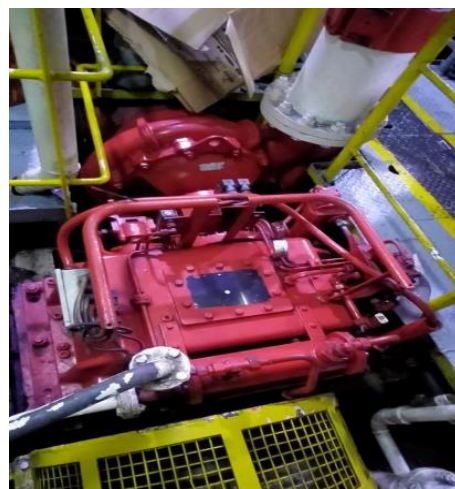
Gambar 2. 2. Fire Fighting Pump
