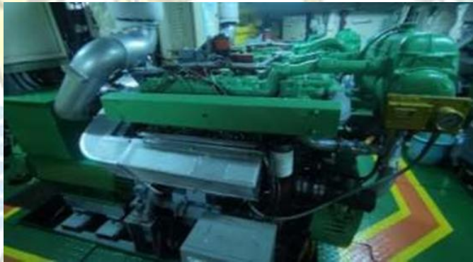
Gambar 2. 3 Diesel Generator Sumber : MV. MERATUS SIBOLGA
