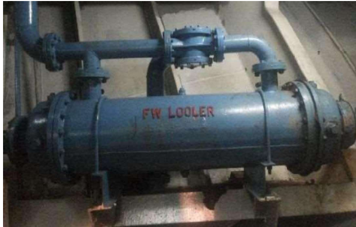
Gambar 2. 8 Fresh Water Cooler
