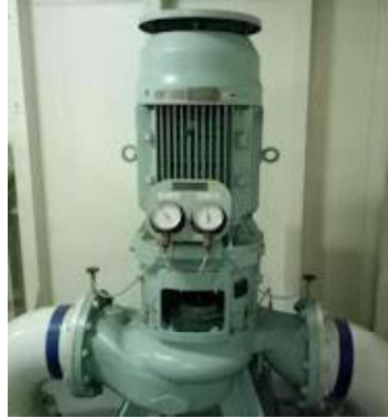
Gambar 2. 12 Pompa Fresh Water
