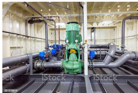
Gambar 2.2 Pipa Air Ballast
