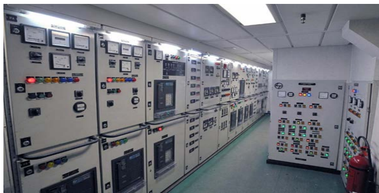
Gambar 2. 1 Engine Control Room
